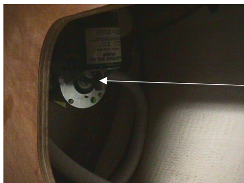
Picture 1 Under Head Sink
