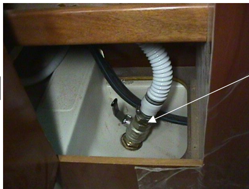
Picture 2 Under Head Sink
