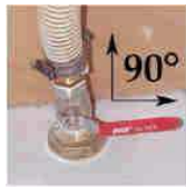
Thru-hull fitting closed
