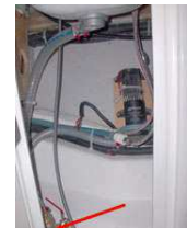
Washbasin draining - Washroom
