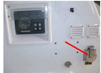
Shore power socket 220V - 30A
