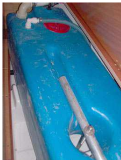
Water tank- To starboard
