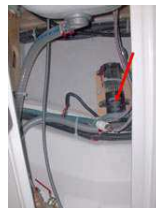
Draining pump for shower
