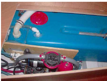
Water tank - To port
