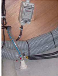
Breaker 32A - Cockpit locker
