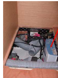
Battery charger - 40A Starboard aft cabin
