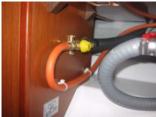
Supply valve - Gas
