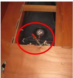
Supply valve Tank (Ref 1)
