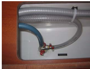
Seawater inlet / House water
