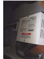
Relay box Location: Starboard saloon
