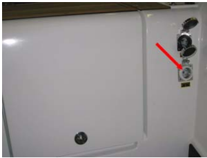
Shore power socket - Aft quarterdeck
