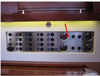
Location: Electrical panel
