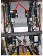
Seawater pump - 24V Saloon
