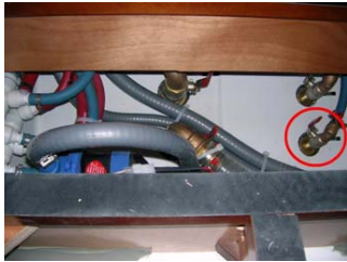
Seawater inlet - Under galley floor
