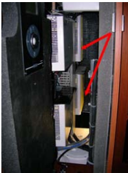
Location: Passageway Power: 2 x 60A
