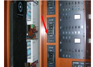
Master switch shore power or generator Location: Port passageway
