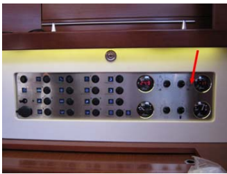
Location: Electrical panel
