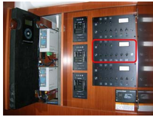
Breaker 220V Location: Port passageway
