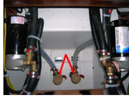
Seawater inlet + Filter
