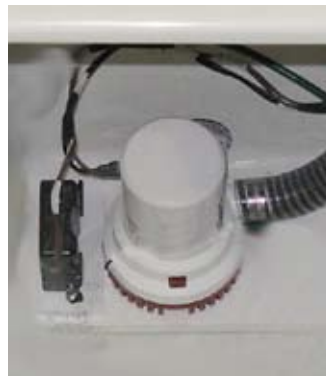
Mid Bilge Pump
