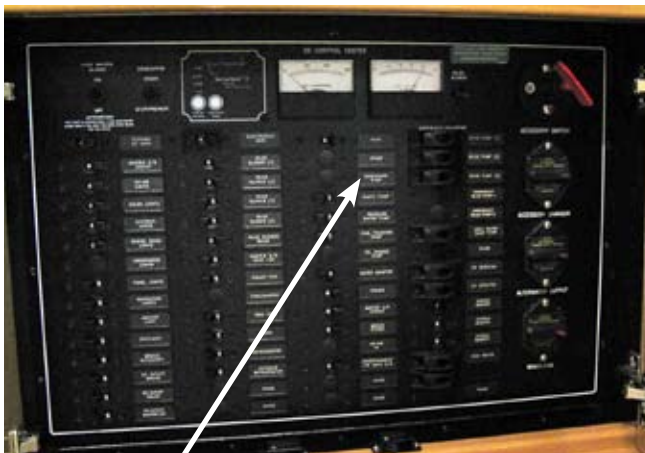
Waste Pump Breaker
