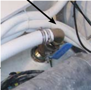
Waste Discharge Valve (Shown Open)
