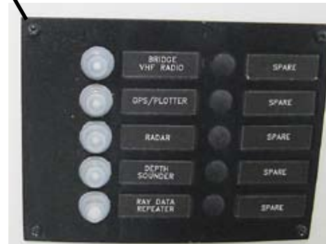
DC Helm Control Panel
