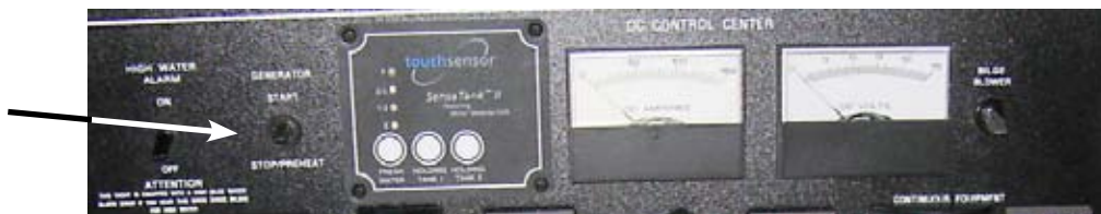
Generator Start Switch DC Panel
