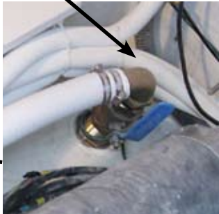
Waste Discharge Valve (Shown Open)
