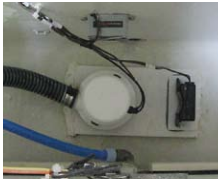
Fwd Bilge Pump
