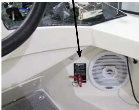
Manual access at helm
