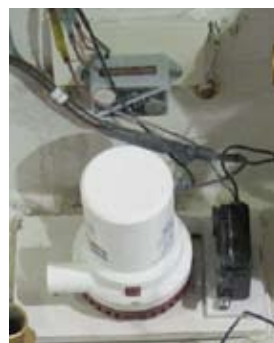
Aft Bilge Pump
