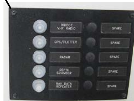
DC Helm Control Panel
