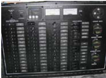
High Water Alarm Switch
