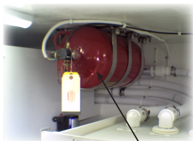
Typical Fire Suppression Tank (54 V Similar)
