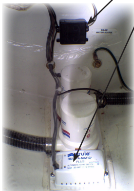
Typical Aft Bilge Pump - 54 Voyager Bilge Similar
