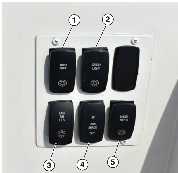
Figure 7-37 – Aft Switch Panel
