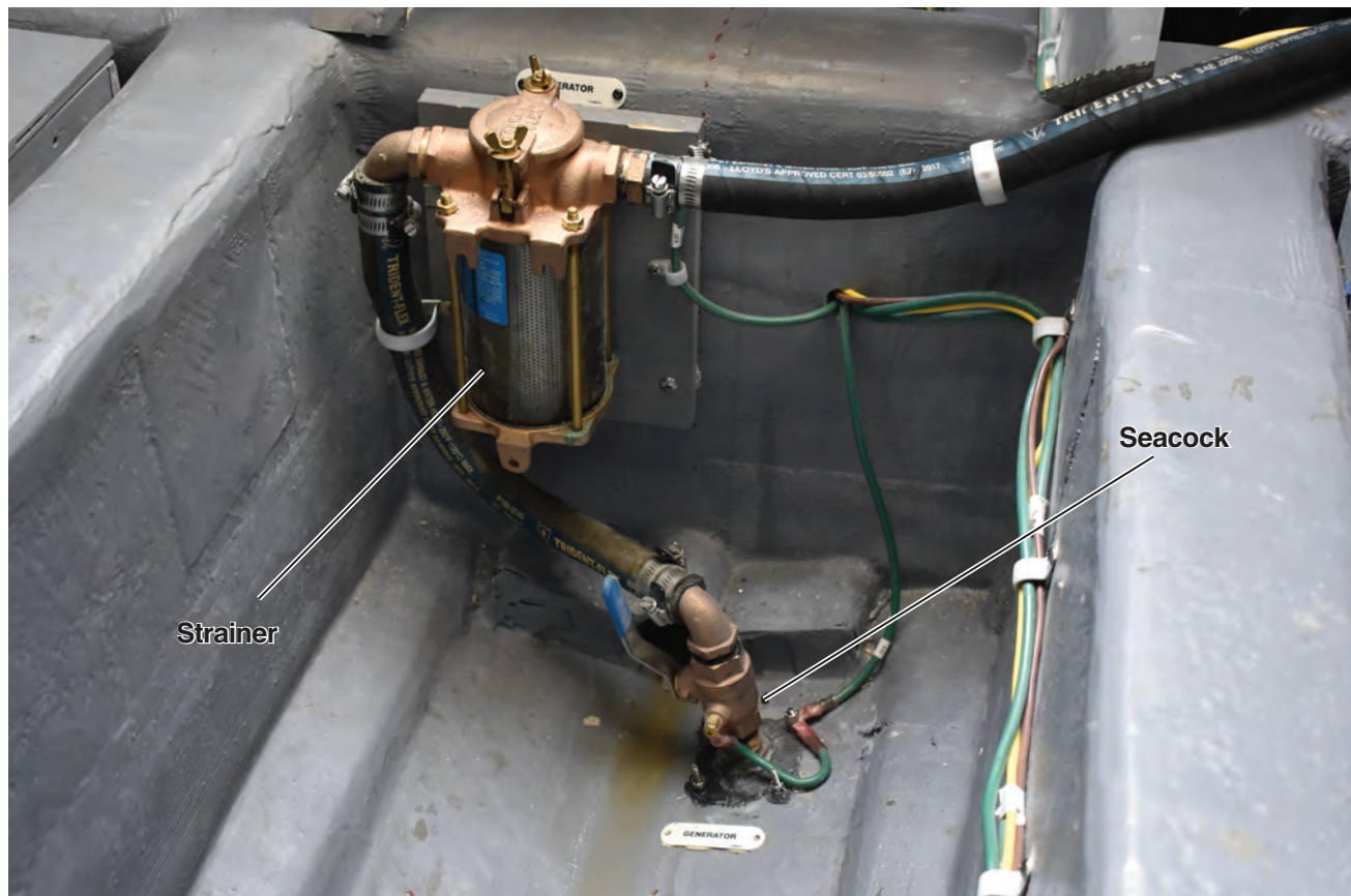
Figure 7-15 – Generator Seawater Strainer and Seacock
