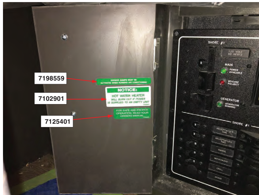
Figure 2-6 – Labels Placed at AC Panel
