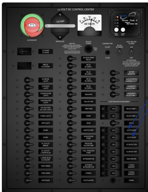
DC CONTROL PANEL
