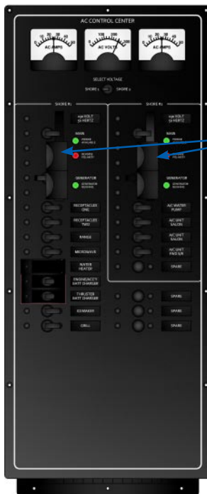
AC CONTROL PANEL
