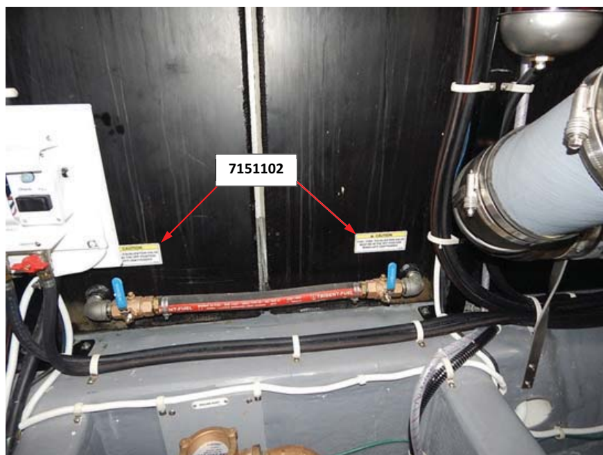
Figure 2-17 – Fuel Equalization Labels on Fuel Tanks
