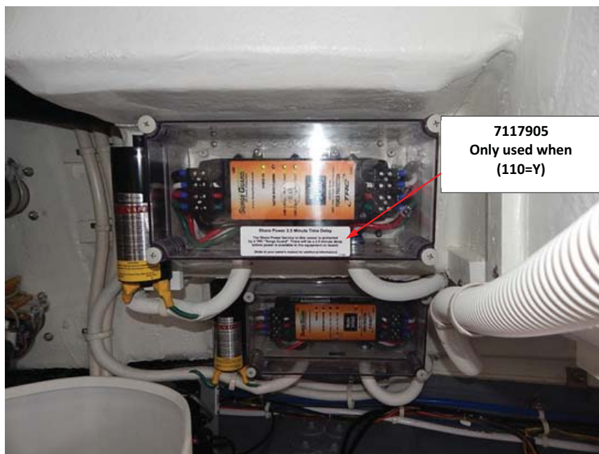
Figure 2-18 – Surge Guard in Engine Room
