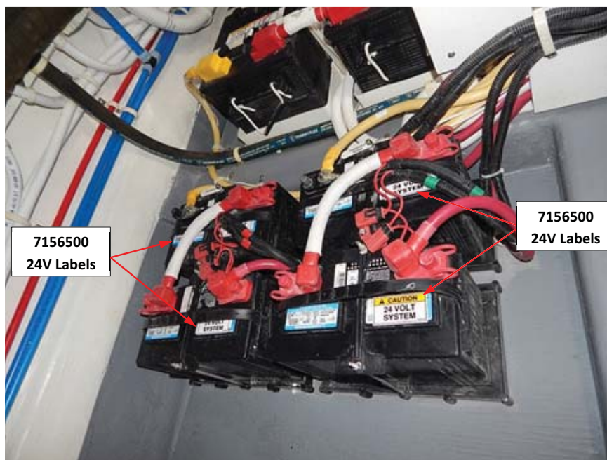
Figure 2-19 – 24-volt Labels on Engine Batteries (1 on Each Battery)
