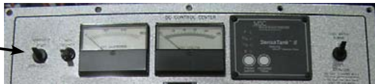
Generator Start Switch
