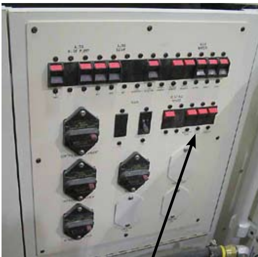
Waste Pump Breaker
