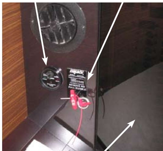
DC Control Panel (door closed)
