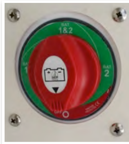
Battery Switch in the “off” Position
