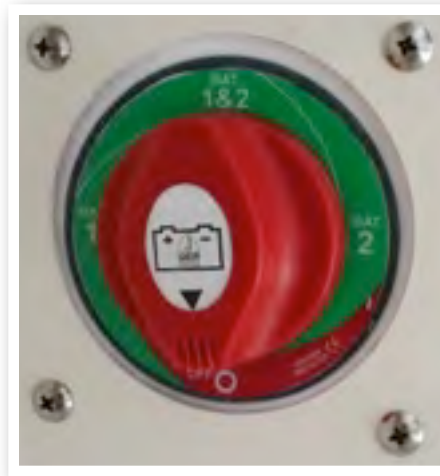
Battery Switch, Shown in the “Off” Position
