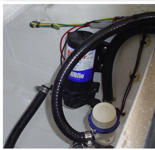
Raw Water Pump
