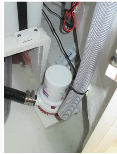
Fwd. Bilge Pump and Float Switch
