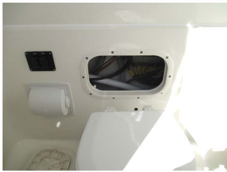
Access to head system valves
