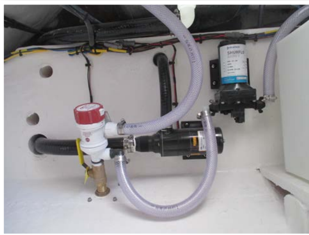
Portside Macerator Pump
