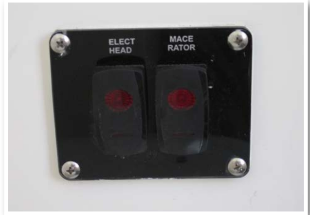
Toilet & Macerator Switch Located on the Starboard Aft Wall of the Head Console
