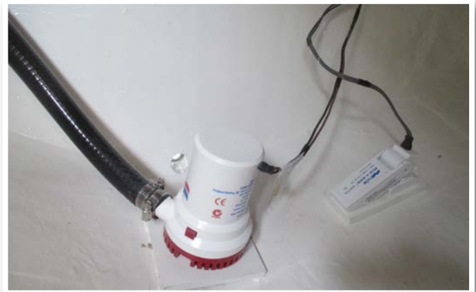
Aft Bilge Pump and Float Switch
