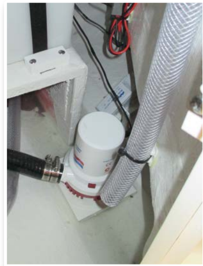
Fwd. Bilge Pump and Float Switch
