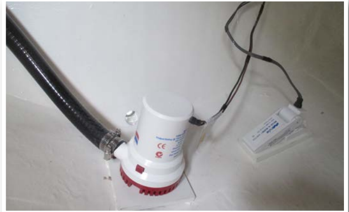
Aft Bilge Pump and Float Switch
