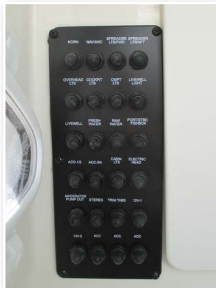
Main Breaker Panel
