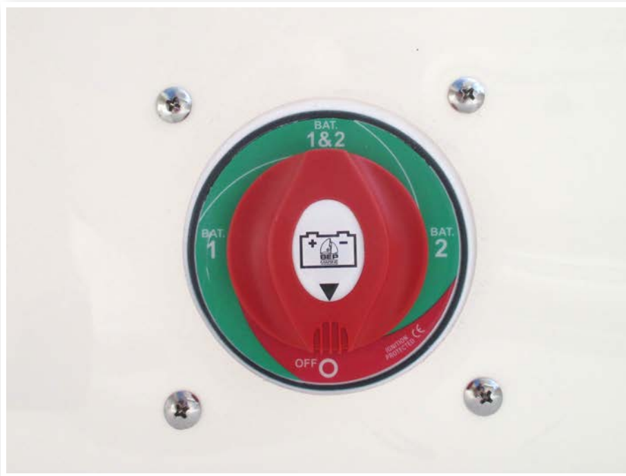
Battery Switch, Shown in the “Off” Position
