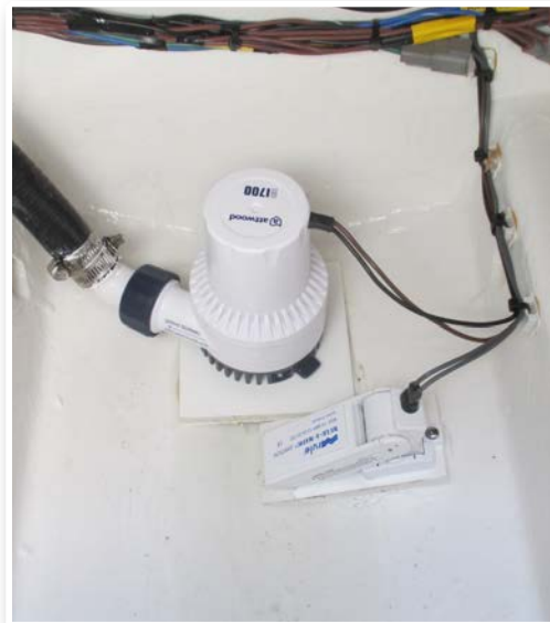
Bilge Pump and Float Switch
