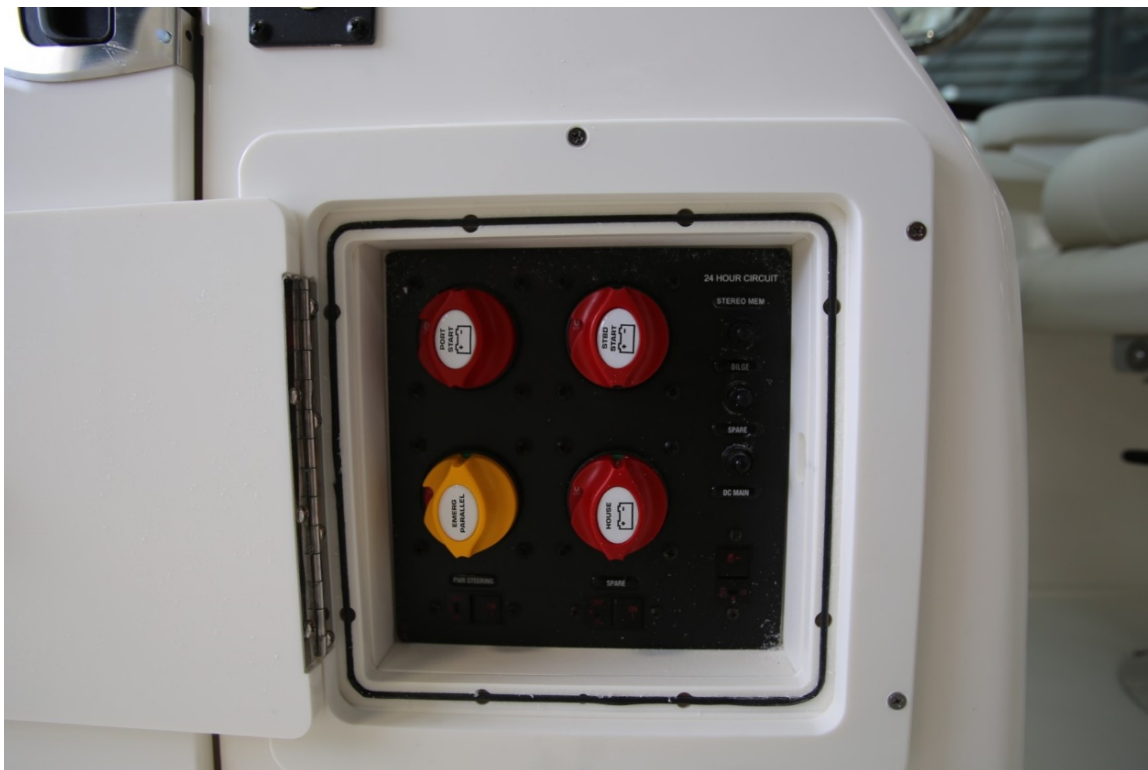
Battery Switch (Shown In Off Position)
