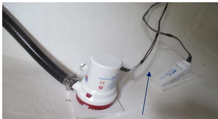
Bilge Pump and Float Switch
