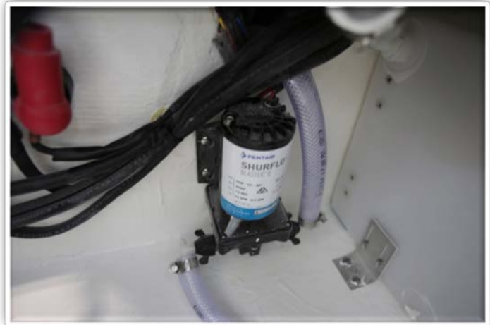
Raw Water Pump
