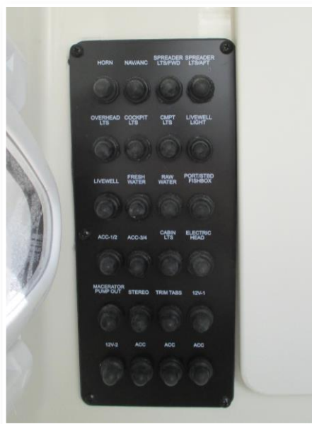
Main Breaker Panel
