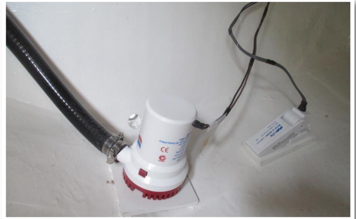
Aft Bilge Pump and Float Switch
