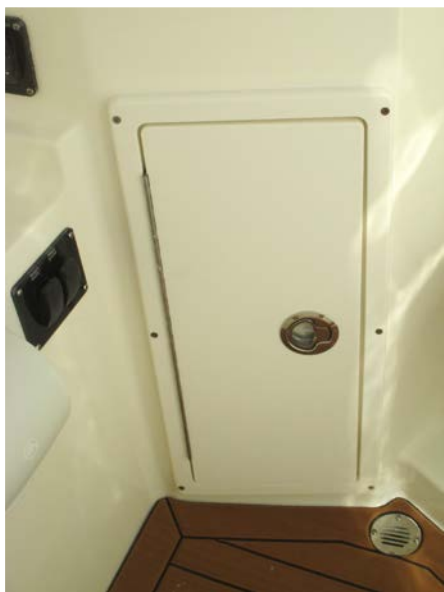
Access to Forward Bilge Area and Head Plumbing
