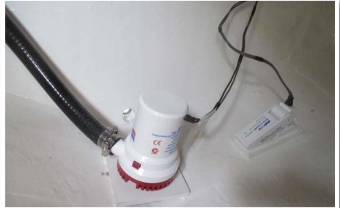
Aft Bilge Pump and Float Switch
