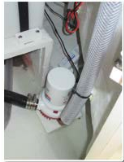
Fwd. Bilge Pump and Float Switch
