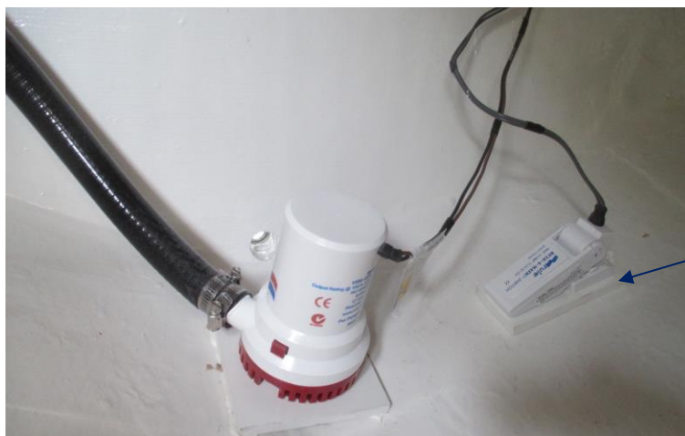
Bilge Pump and Float Switch
