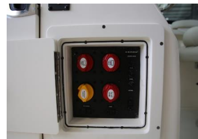
Battery Switch (Shown In Off Position)
