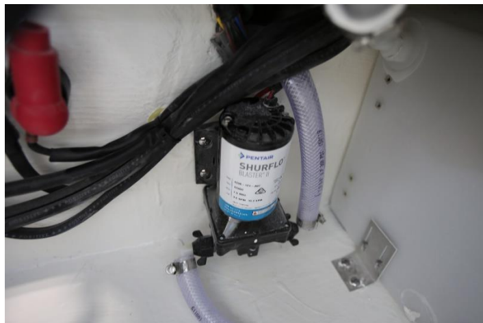
Raw Water Pump
