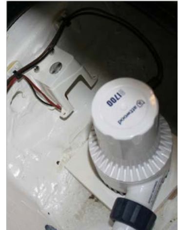
Aft Bilge Pump and Float Switch
