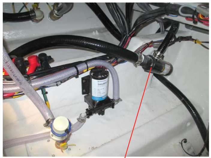
Starboard Macerator Pump
