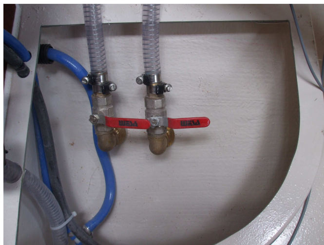
Figure 21: Rapid shut off valve shower room
