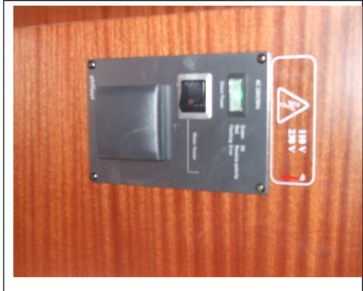
Figure 13: Shore connection panel
