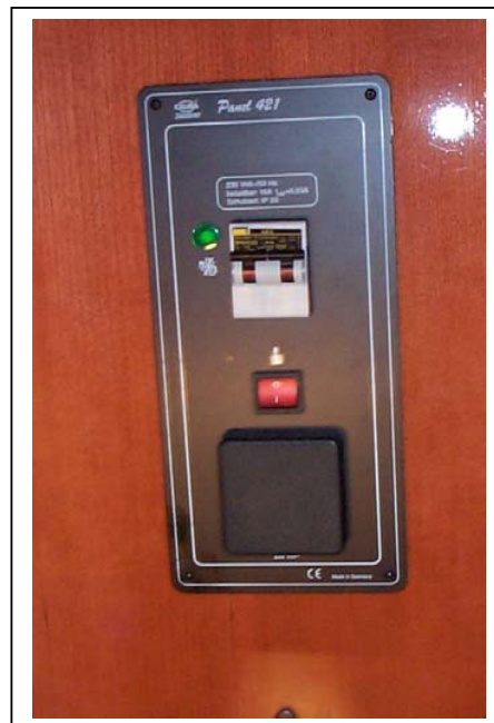
FIGURE.:SHORE CONNECTION SWITCH BOARD
