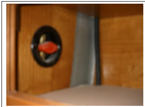
ABB: GAS SHUT-OFF VALVE
