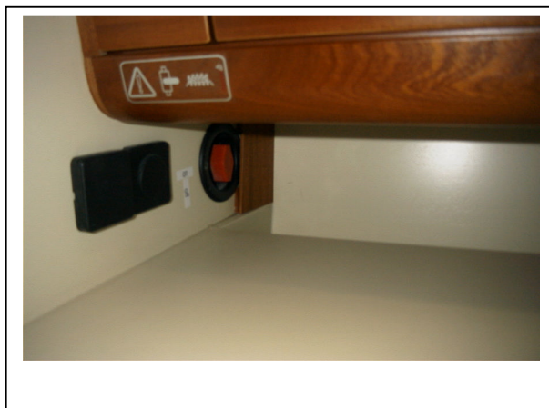
ABB: GAS SHUT-OFF VALVE
