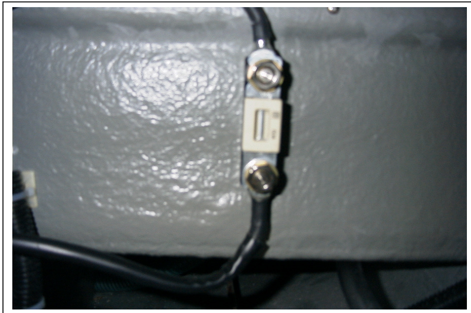
ABB.: MAIN FUSES
