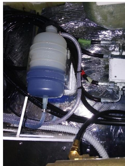
Cooling tank filled 1/3
