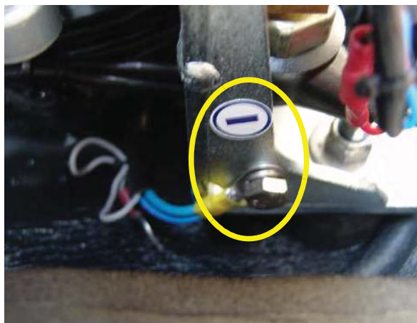
Fig. A.3.6-3: Connection starter battery minus cable
