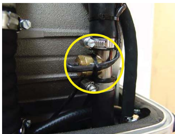
Fig. A.3.7-5: Thermo-sensor raw water out
