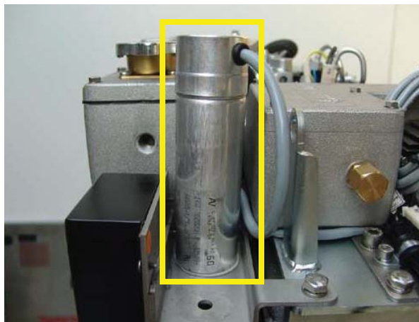
Fig. A.3.6-20: Booster capacitor 230V/50Hz
