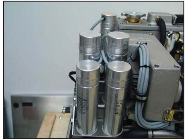
Fig. E.4.1-1: Discharge capacitors
