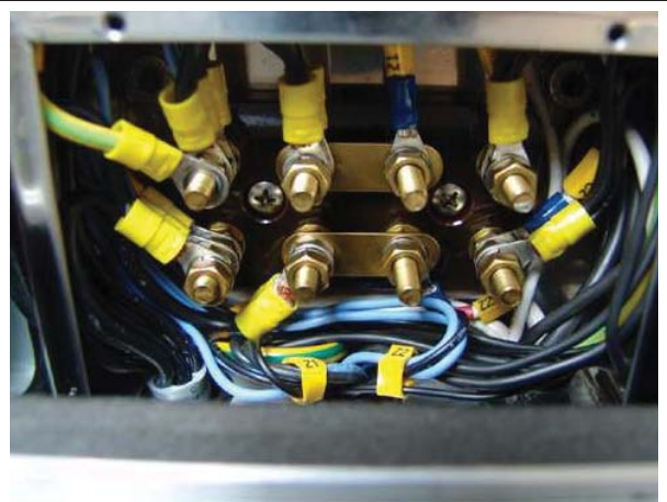
Fig. A.3.6-13: Generator power terminal box 120V/60Hz
