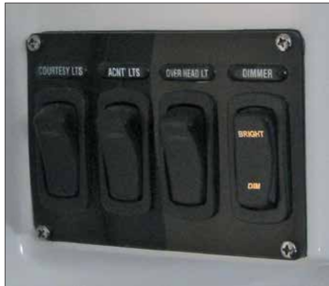
Cabin Switch Panel
