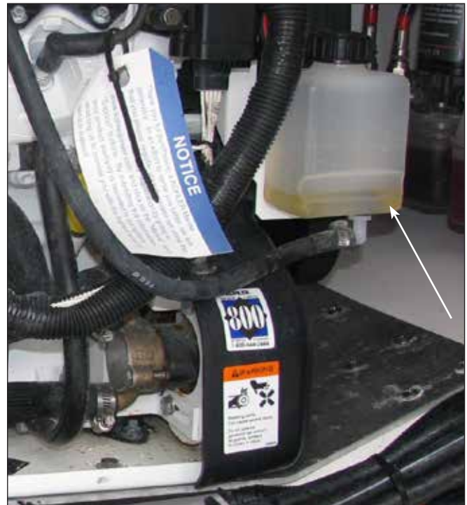
Generator Coolant Recovery Tank
