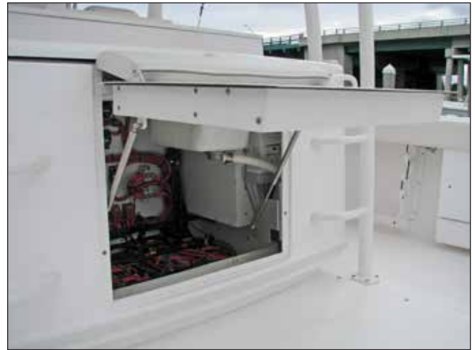
Electrical Systems Compartment Hatch
