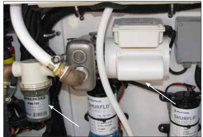
Air Conditioner Seawater Pump & Strainer
