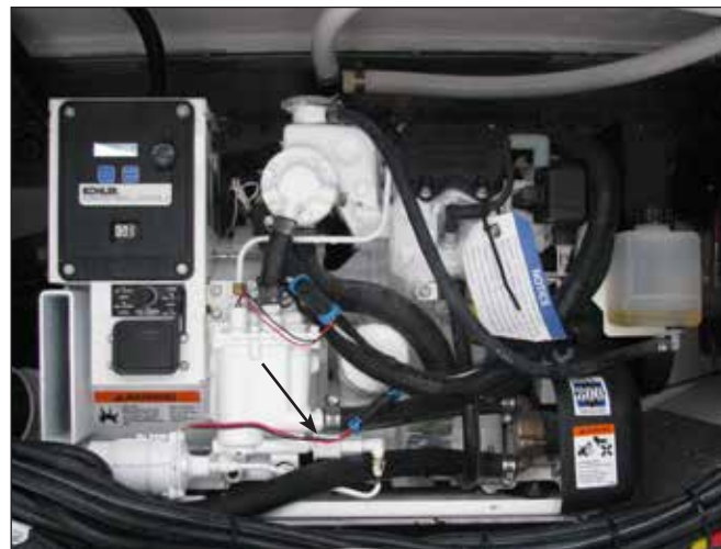
Generator In-Line Fuel Filter
