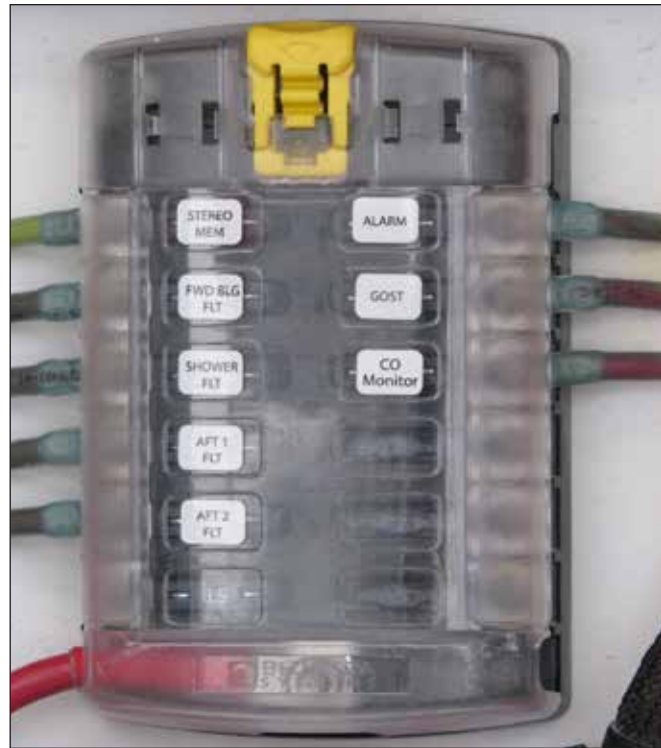
Continuous Power Fuse Panel
