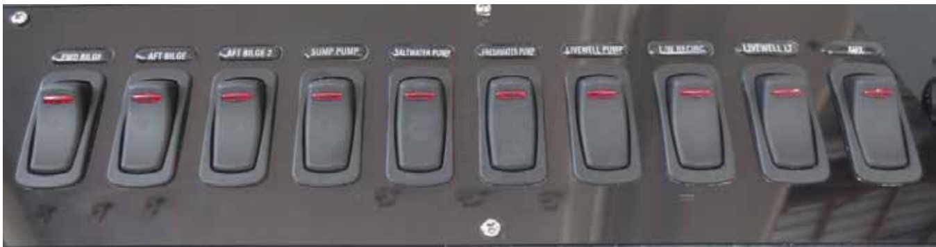
Starboard Helm Accessory Switch Panel
