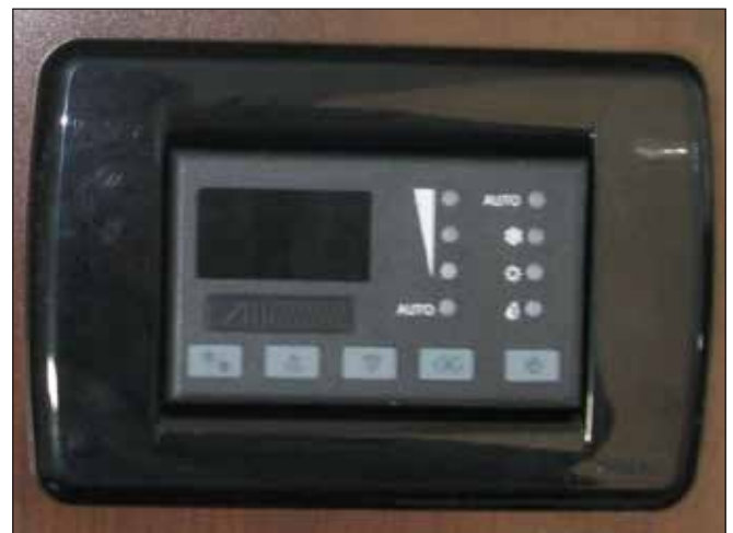
Air Conditioner Control Panel
