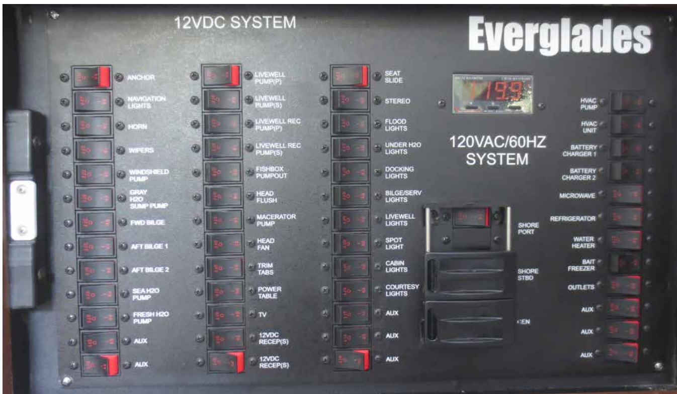
Cabin DC/AC Panel
