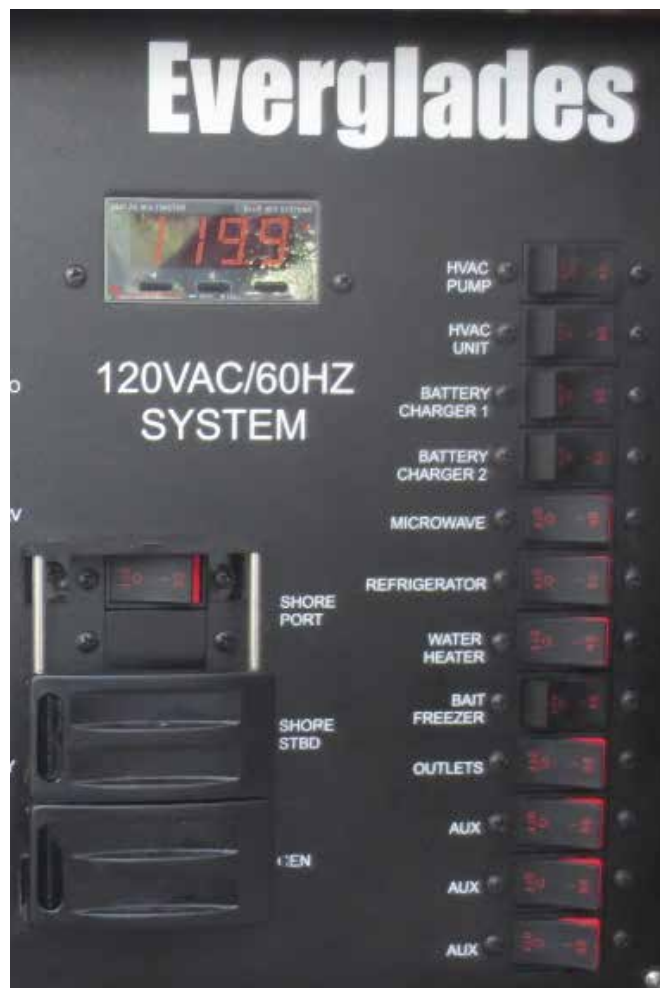
Shore PWR/Generator Main Breakers
