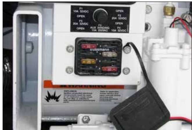
Typical Generator Fuse Panel
