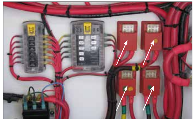
Typical Helm Master Heavy Duty Main Fuses
