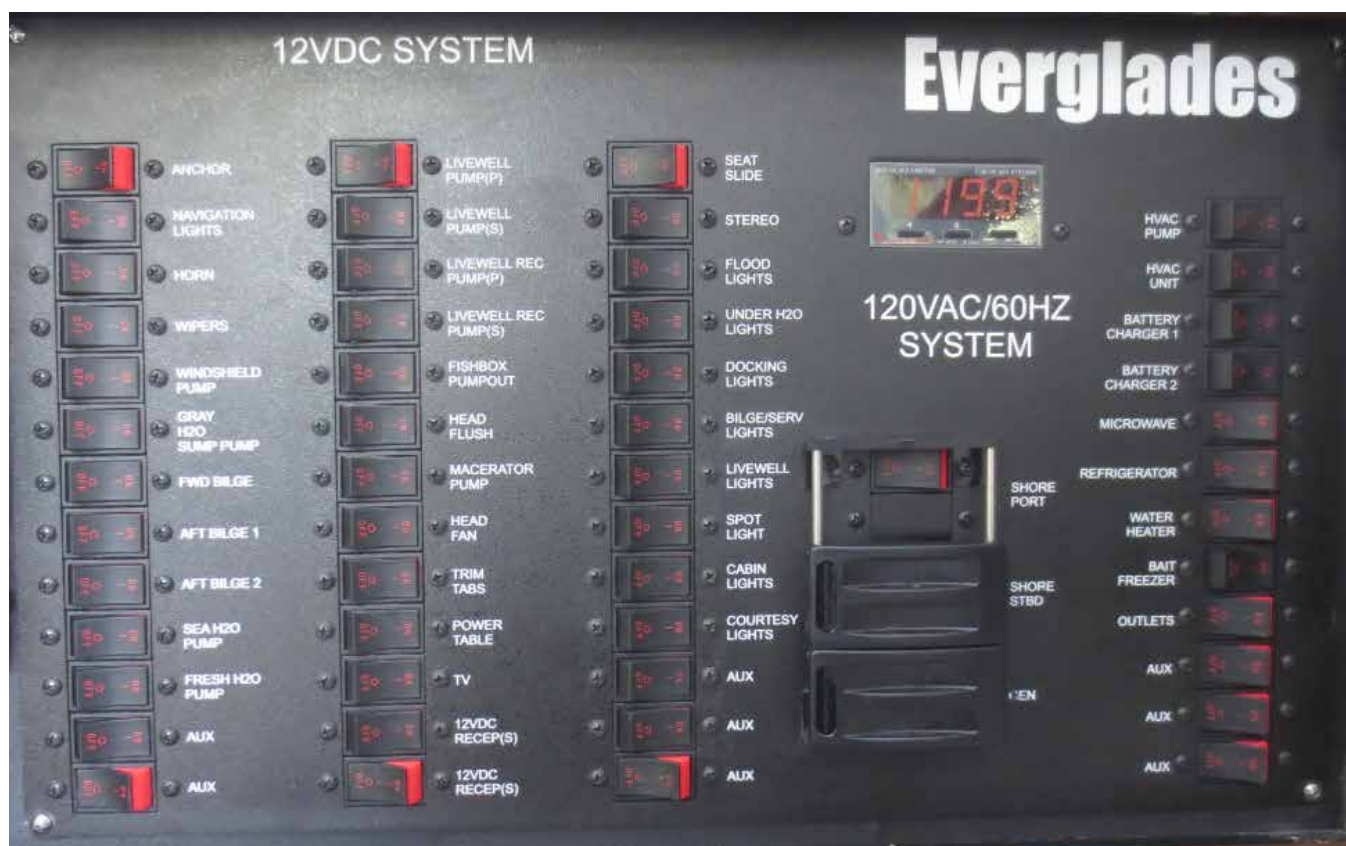
Cabin DC/AC Panel
