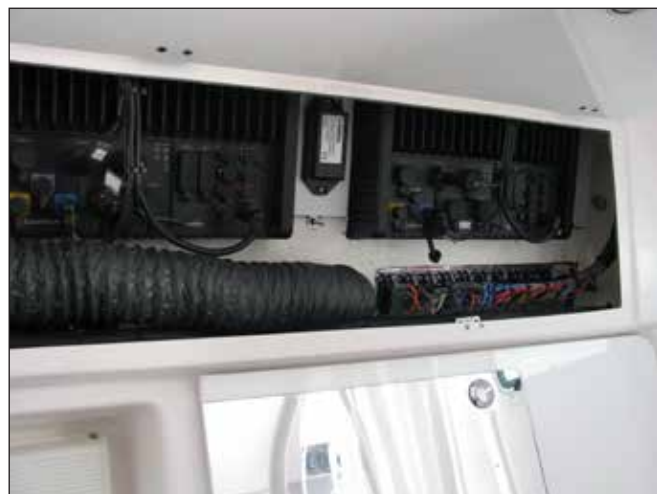
Electronics Access in Rear Cabin Bulkhead
