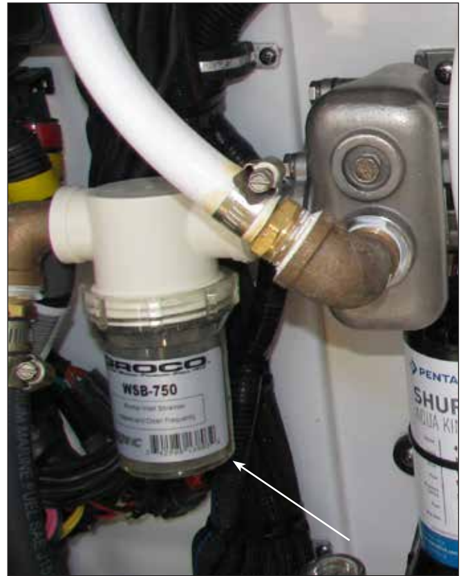
HVAC Pump Sea Strainer
