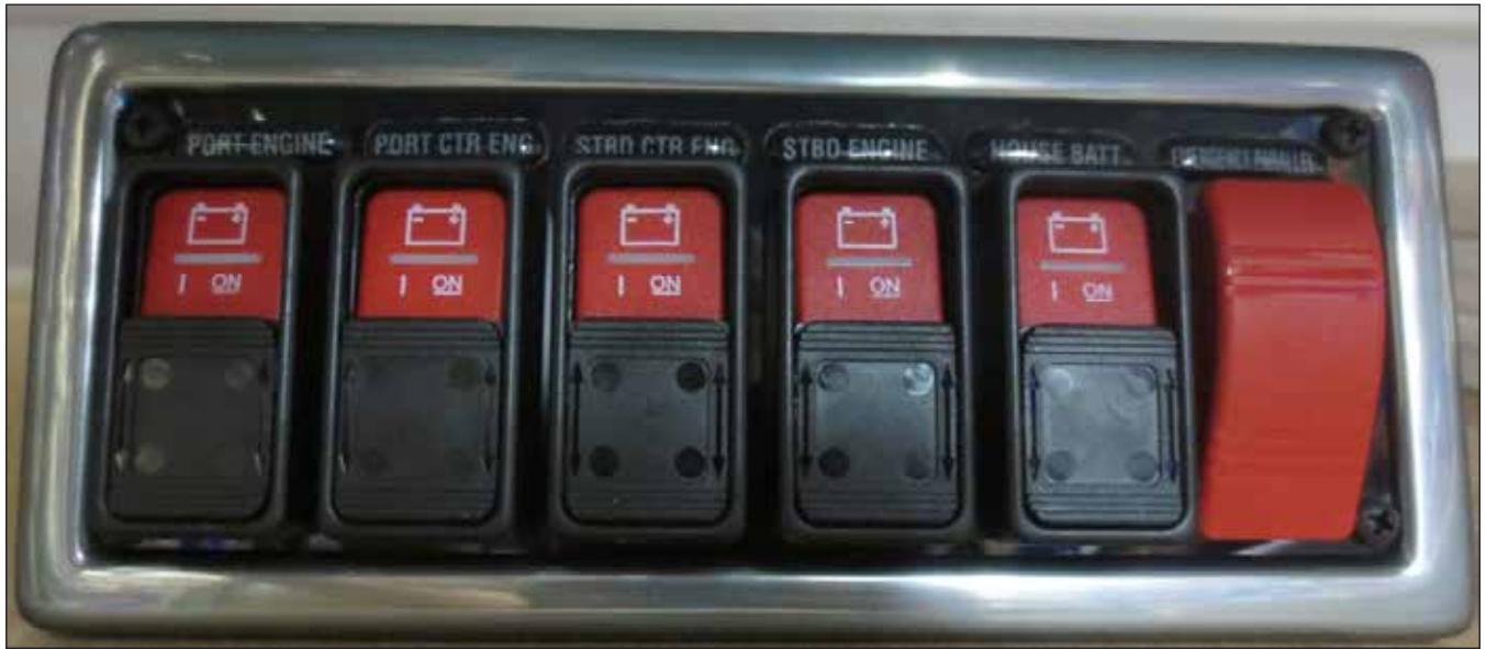
Battery Switch Panel at Helm
