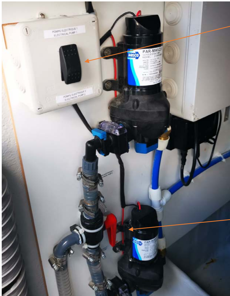
Selector switch for freshwater pumps
