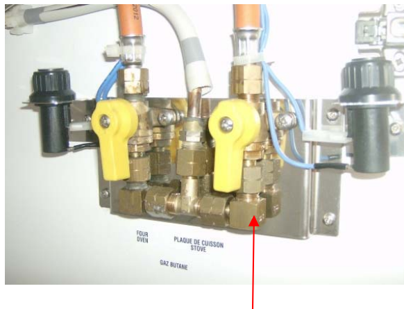
Gas shut off valves under sink
