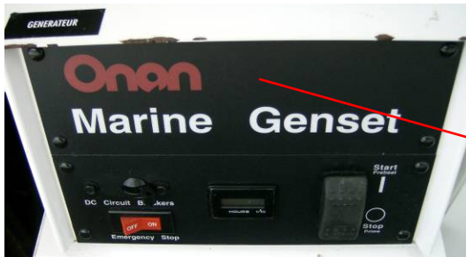
Main breakers for the generator
