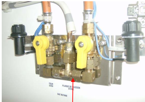
Gas shut off valves under sink
