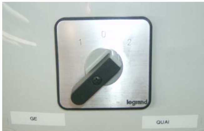
Generator (GE) / Shore power (QUAI) selector switch
