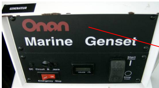
Main breakers for the generator
