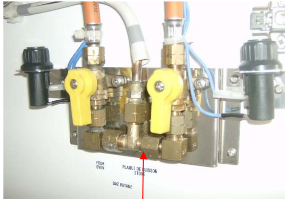
Gas shut off valves under sink
