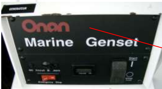
Main breakers for the generator
