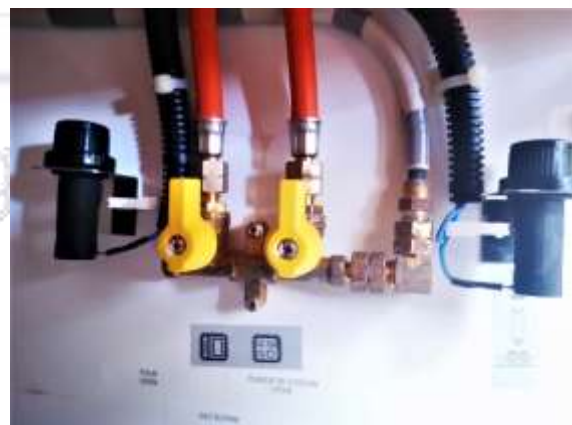
Propane shut-off valves
