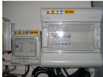
Control panel 220V
