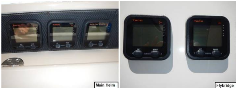
All engine instruments are Yamaha digital multi functional gauges. Gauges functioned properly with all engine status information being displayed. (Photo's were not taken of the gauges powered up as they do not photograph well in the sunlight.)
