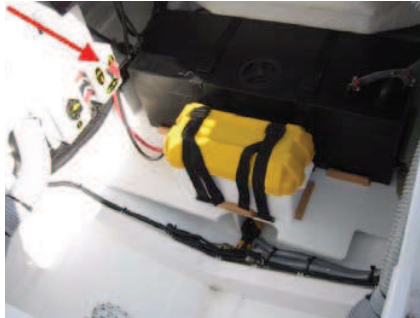
Location: Cockpit locker
