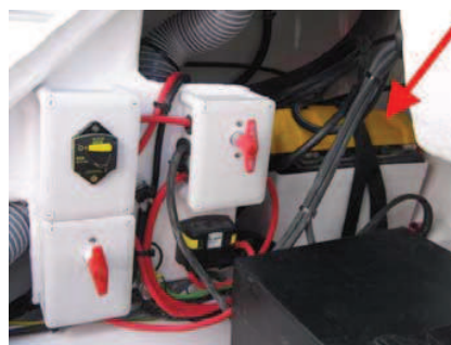
Service battery: 110A
