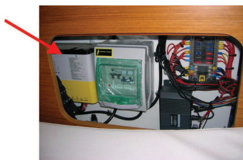
Battery charger Location: Cabin
