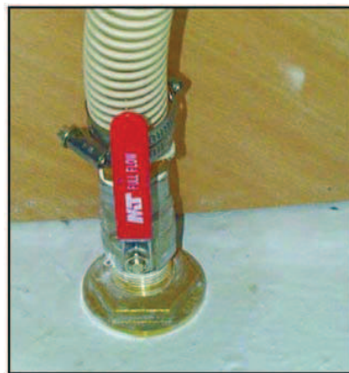
Thru-hull fitting open
