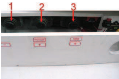
Battery switch Location: Cockpit locker
