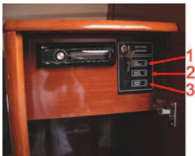
Battery switch control Location - Starboard saloon
