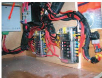
Battery charger Power: 12V 25A Location - Aft cabin
