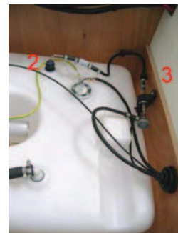
Joining - Diesel (Ref 2) Diesel pump (Ref 3)
