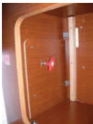
Remote pull switches (Ref 1)
