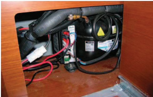
Refrigeration unit Location: beneath the TV unit
