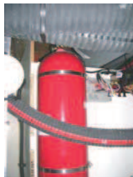
Fixed extinguisher (Ref 2)
