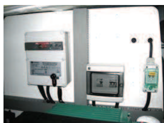
AC Source selector Differential circuit breaker Bipolar circuit breaker - House
