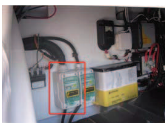
Breaker - Protection (Reference 2)
