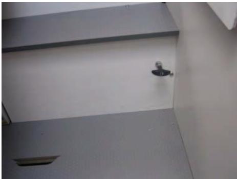
Remote pull switches - Supply tanks (Ref 3)
