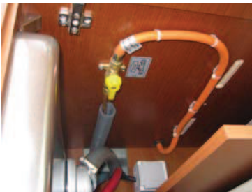
Supply valve - Gas Location: Under the sink
