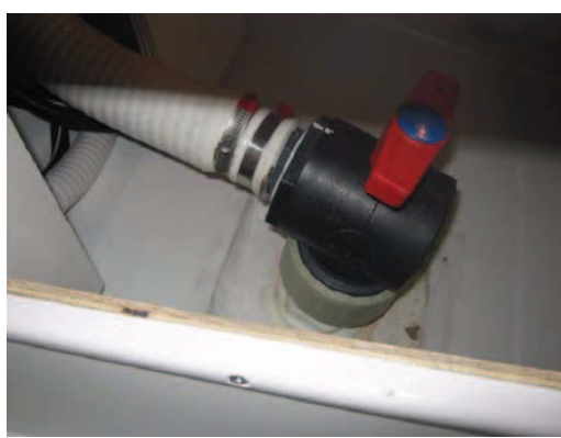
WC evacuation Location: Technical room
