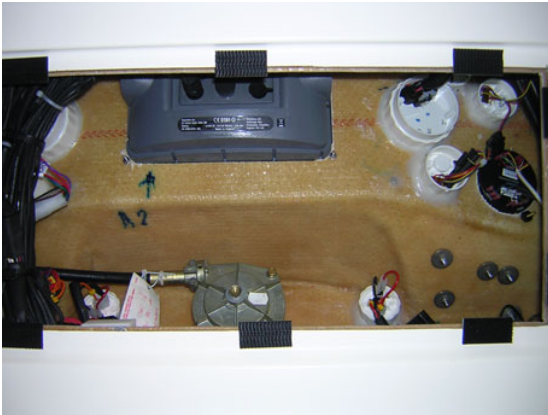
Access to the control panel connections
