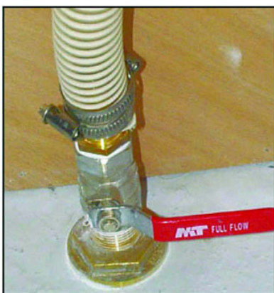
Thru-hull fitting closed
