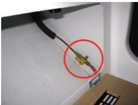
Gas supply valve
