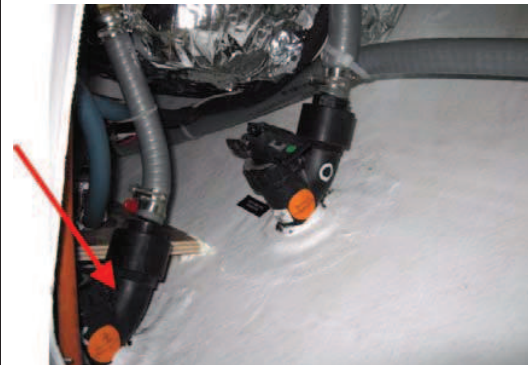
Sea water intake
