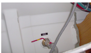
Seawater inlet - Under Washbasin
