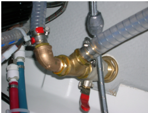
Drainage - Washbasin + Washroom shower
