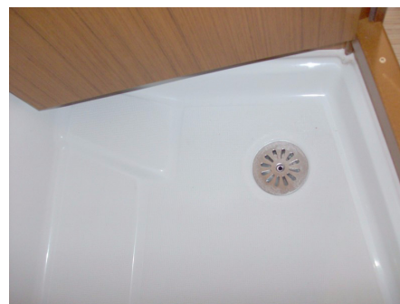
Drain plug shower draining
