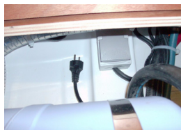
Water heater - 220V socket
