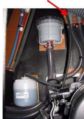
Location: Engine compartment
