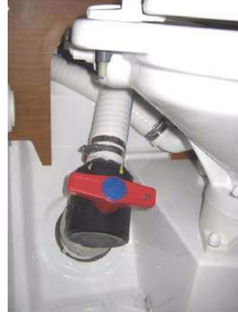
WC evacuation gate valve to sea
