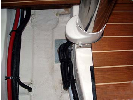
Mast harness exit at the stanchion base
