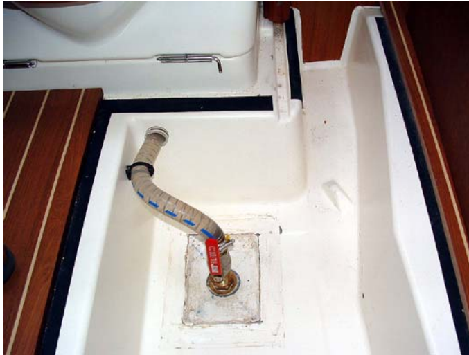
Thru-hull fitting with engine water inlet valve
