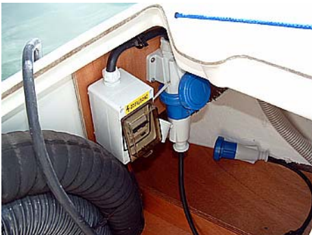
Shore power socket
